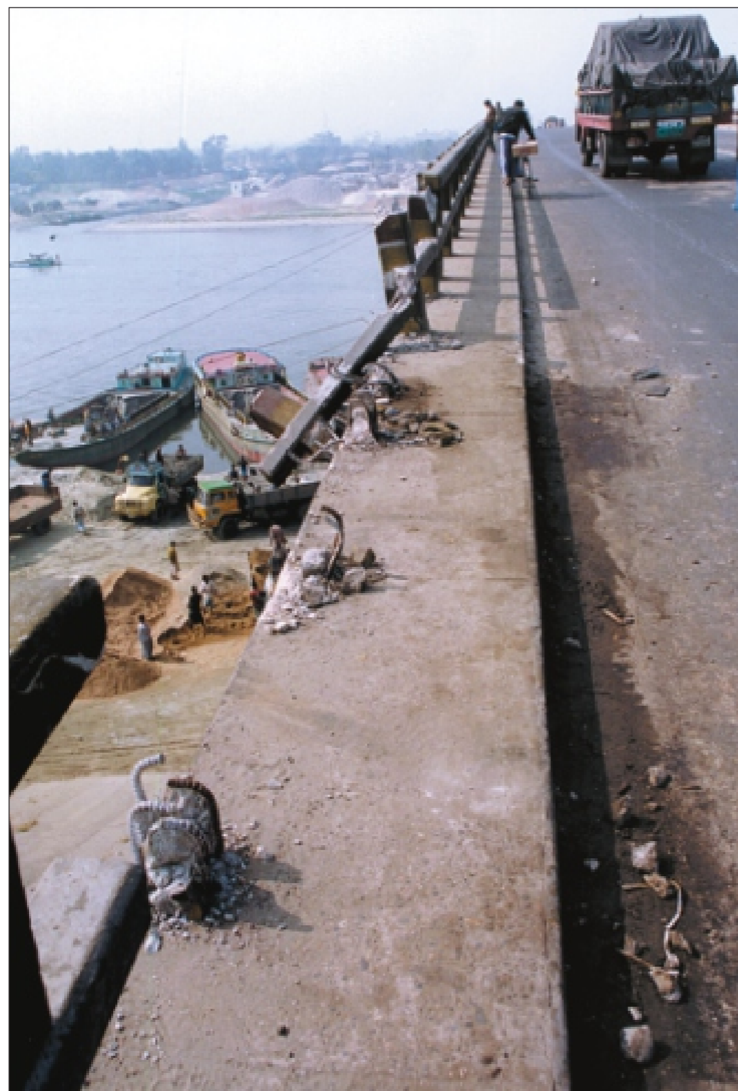
The Kanchpur Bridge on the river Shitalakhya remains in such a dilapidated condition with broken railings. Hundreds of vehicles cross the bridge every day risking the passengers' lives.
