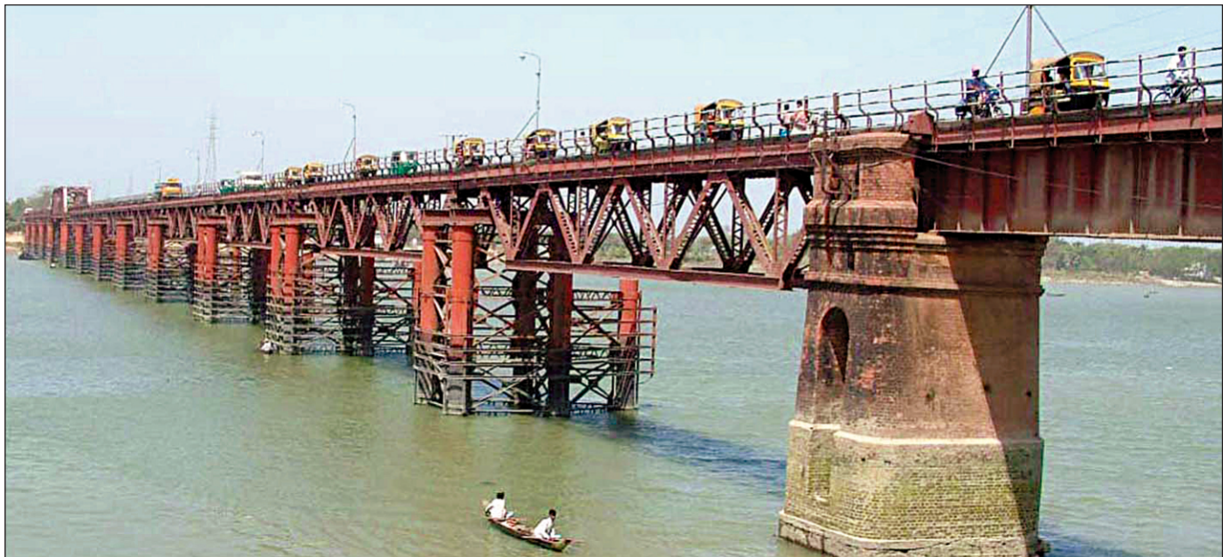
Renovation of the century-old Kalurghat Bridge is going on (top) and a view of the bridge before the renovation work (bottom).
