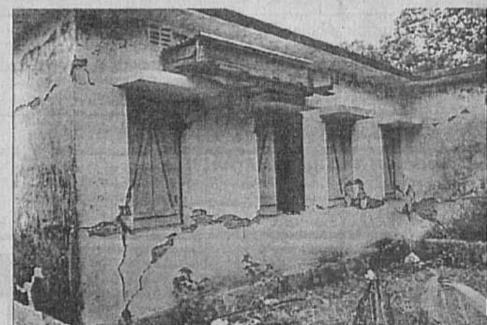
Severe damage to brick masonry building in Kolabunia during July 2003 Rangamati-Barkal earthquake.
