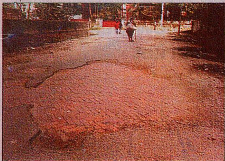
Worn-out roads at Katalganj, left, and Halishahar. The roads go under water during rainy season and accidents are commonplace, but the authorities concerned are indifferent to the problems for years.
