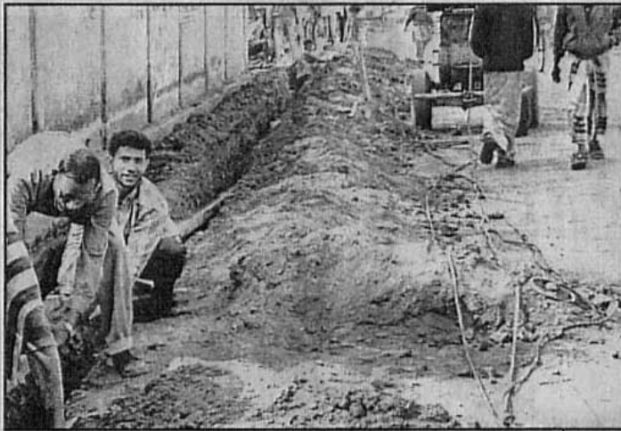
ENTHUSIASM ALL AROUND.. Laying of gas pipeline in Bogra town is going on in full swing. The photo was taken from Badur Tola area on Friday.
