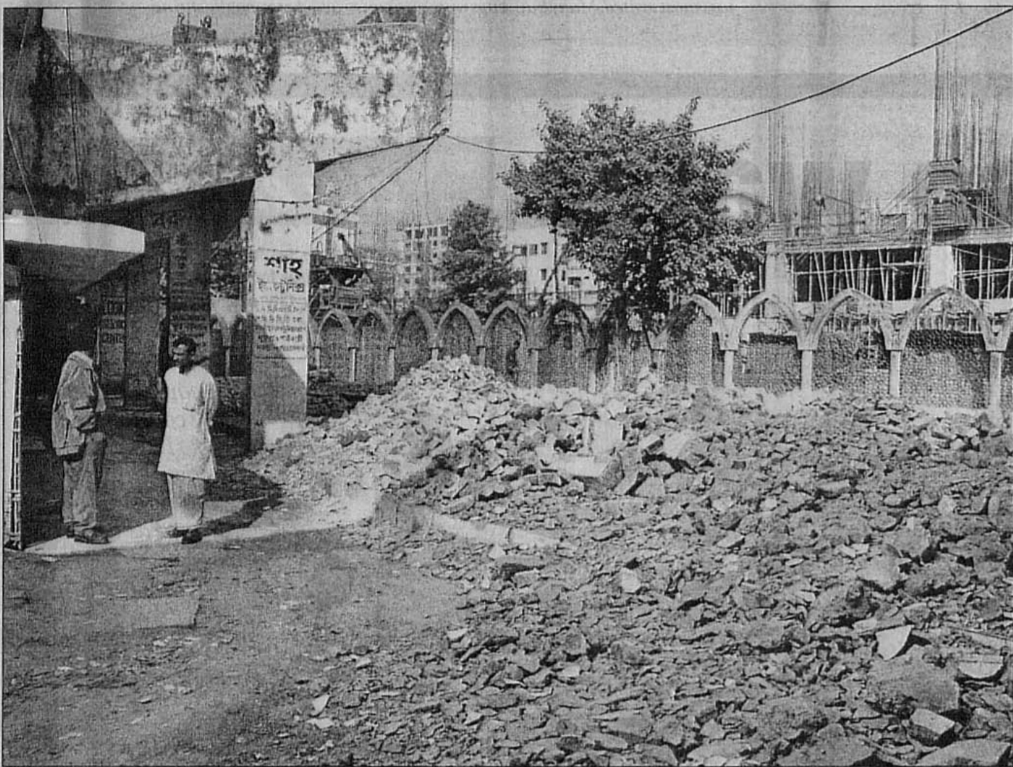
Rubble from the 28 shops that had been illegally built on NSC land awaits cleaning.
