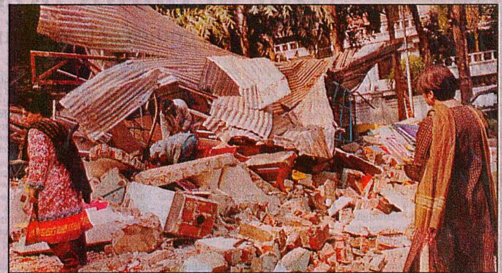
Dhaka City Corporation (DCC) bulldozes the Green Del International School in Gulshan on Saturday evening.
