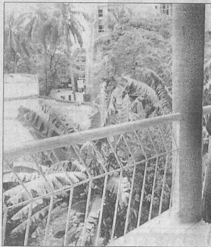
Horizontal bars of railing invite children to climb and cause accident
