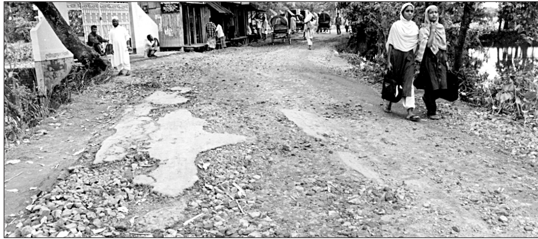
Flood caused by incessant rains has damaged the Tangibari-Munshiganj Road. The unfit road needs immediate repairing.
