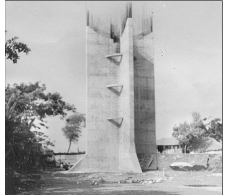
An incomplete overhead tank in Kalapara Pourashabha. Its work started three years back which was abandoned later by the concerned contractors due to reasons unknown to all. Acute drinking water crisis prevails in the area.
