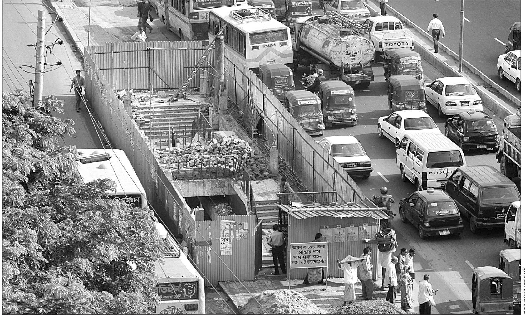
BETTER LATE THAN NEVER: The DCC has started renovating the Karwan Bazar underpass recently.
