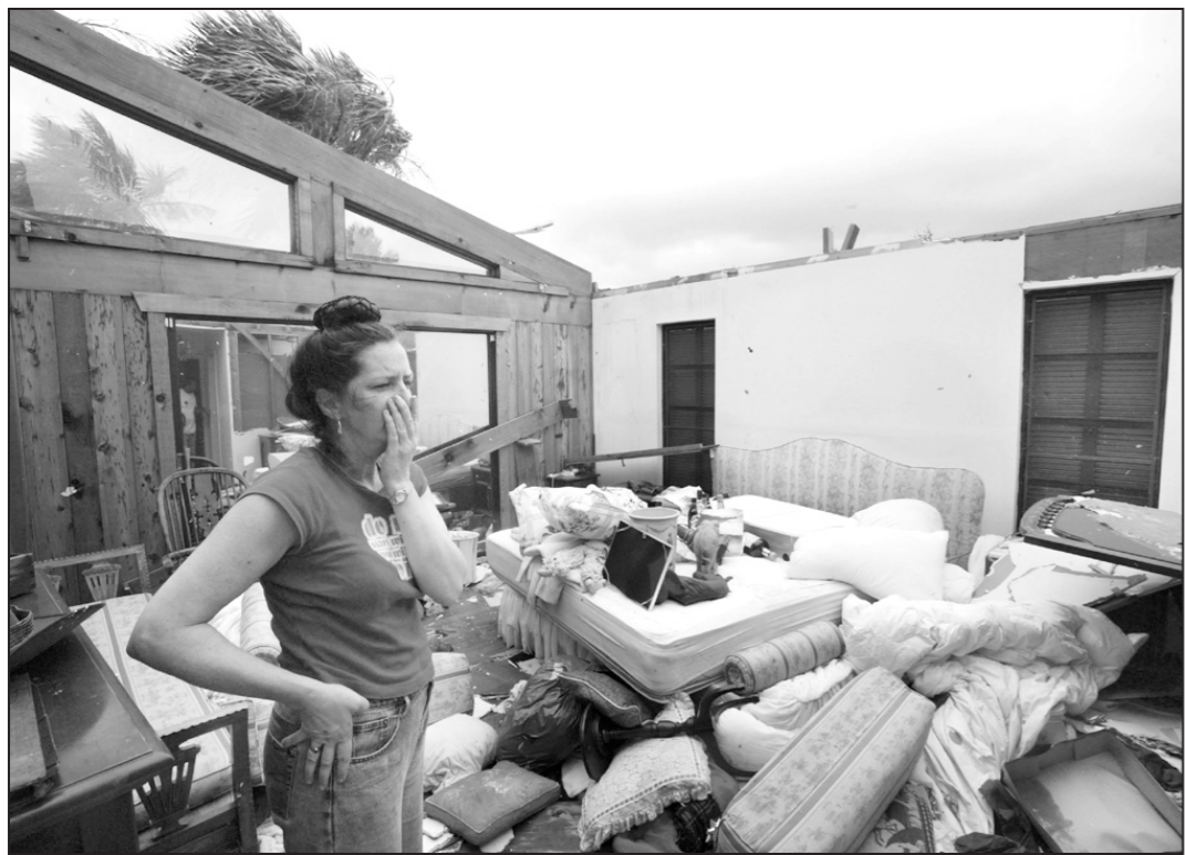
Constance Kenney surveys what is left of her father's bedroom after the home was blown apart by winds caused by Hurricane Jeanne Sunday in Sebastian, Florida. Jeanne, which has been downgraded to a tropical storm, moved across the state of Florida after making landfall the night before.
