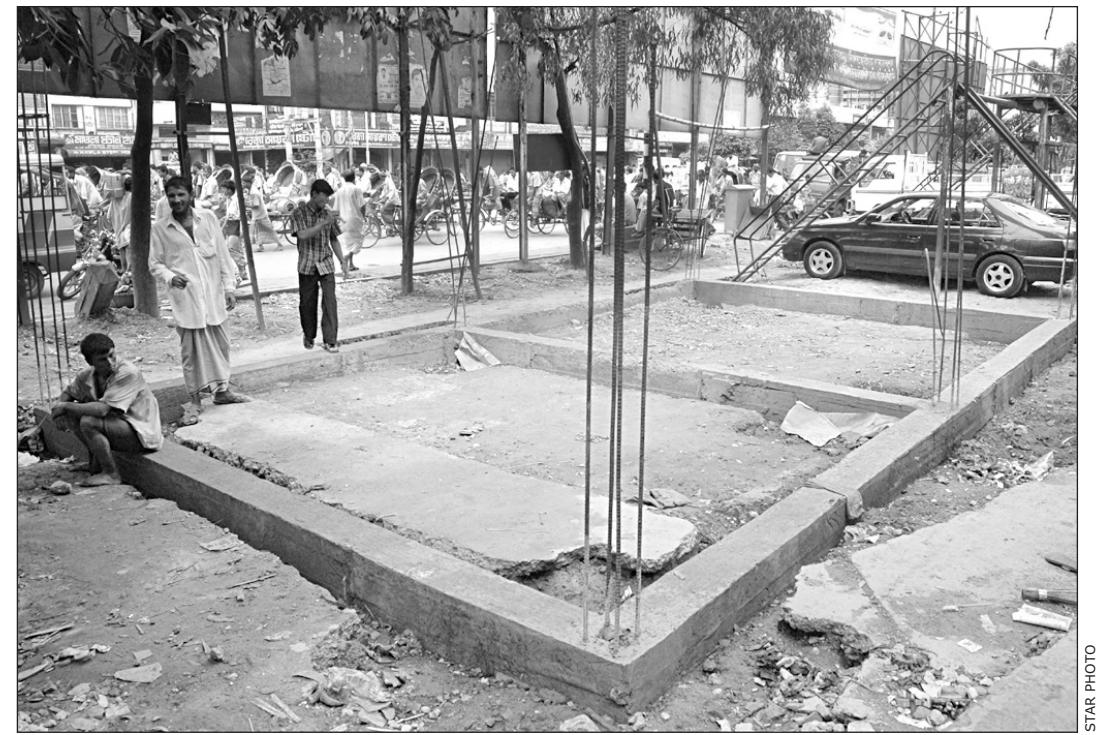
Work on this public toilet is stalled because of a dispute between local commissioners and contractor.
