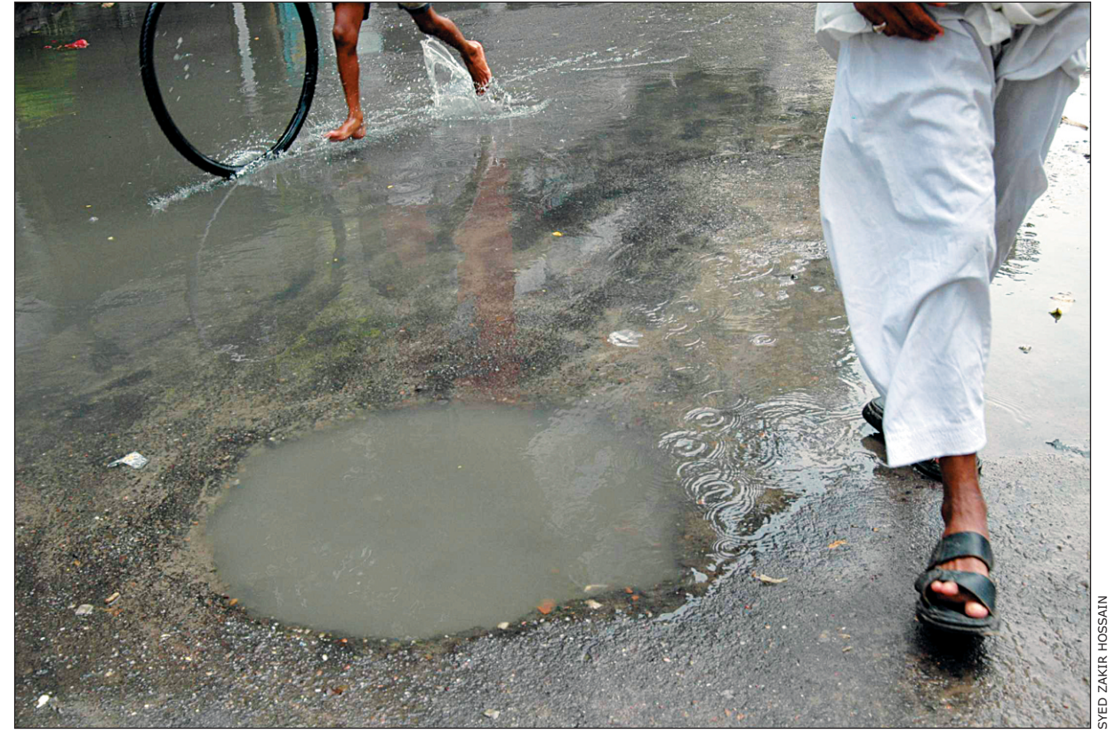
Open manholes in major roads and alleys pose danger to pedestrians and vehicles as well.
