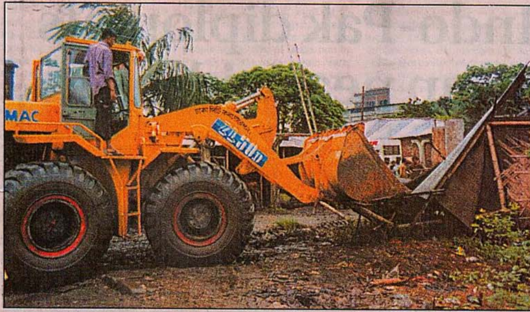
Dhaka City Corporation bulldozed illegal structures at Golapbagh play ground in the city yesterday.
