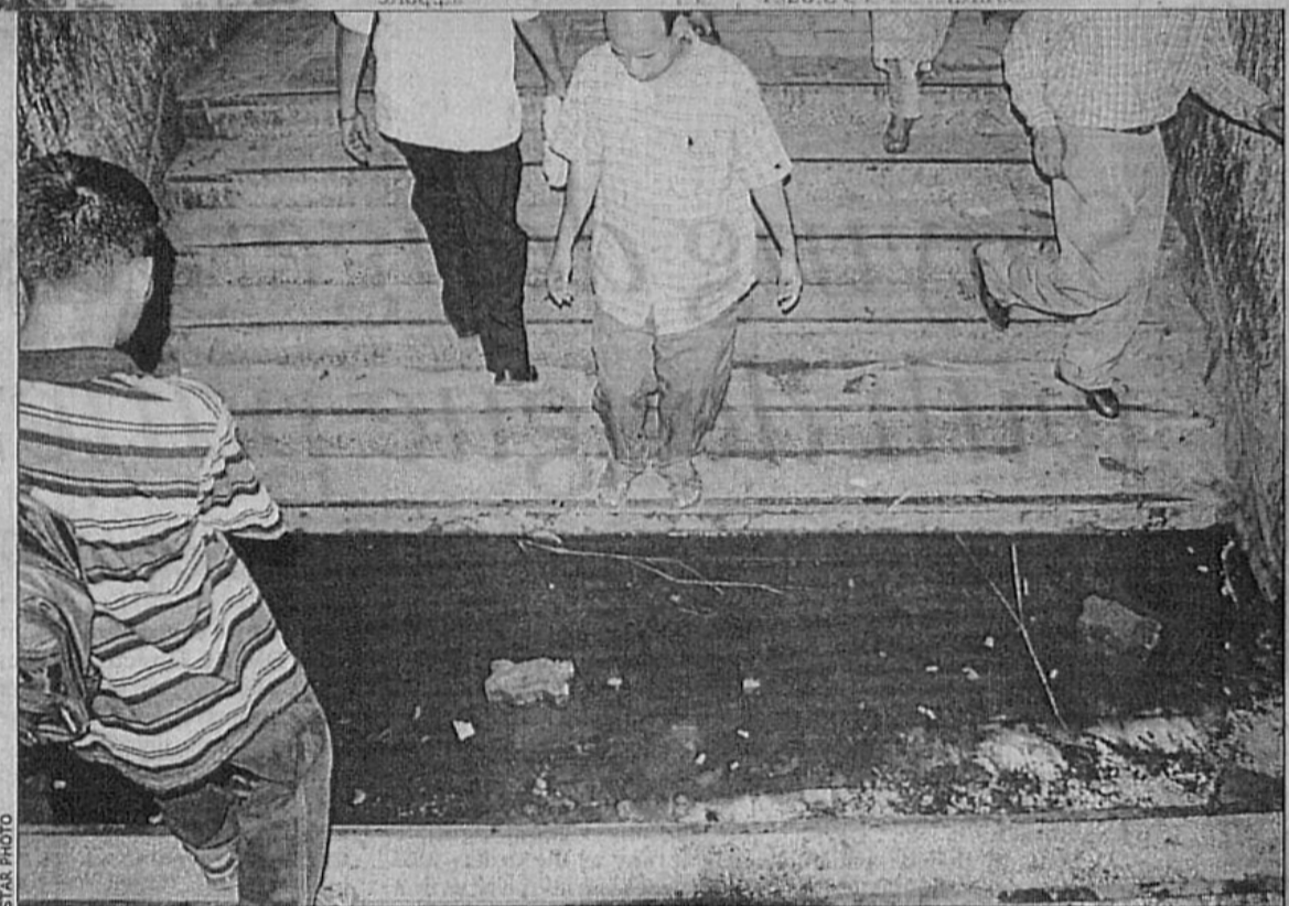
Stagnant water at Karwan Bazar underpass
