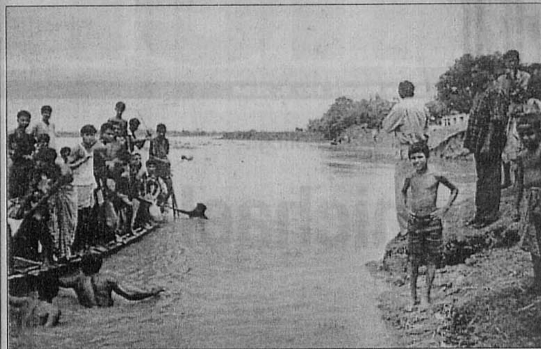
People repairing the erosion-affected bankment of the Bangali river at Balua in Mohimaganj, Gobindaganj upazila.
