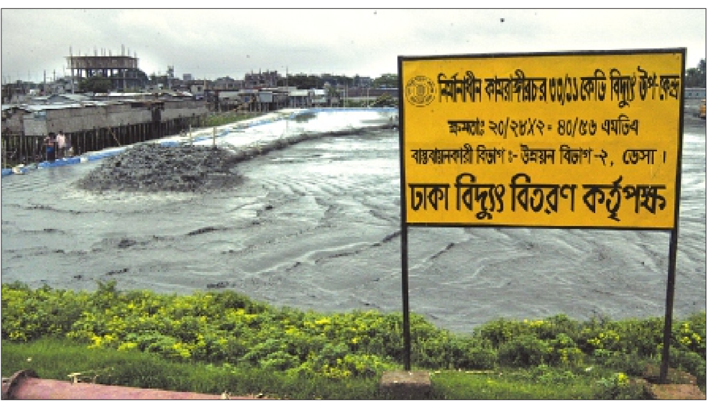
Dhaka Electric Supply Authority has filled up a huge chunk of the wetland by the bank of the river Buriganga to install a power sub-station in Kamringirchar. The stretch of the land has been classified as the shore of the river.
