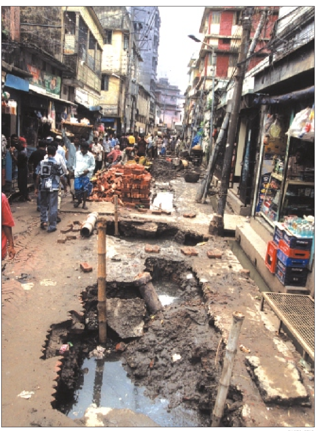
This ravaged road in Becharam Deuri in Old Dhaka, which plays host to accidents, stands as a testament to the mindless digging of roads by the utility agencies.
