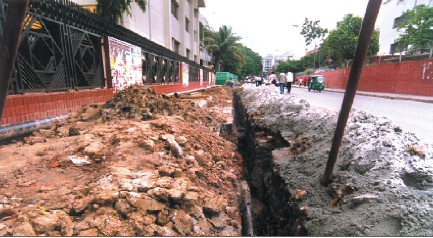
Authorities have dug up the road between Bangladesh Secretariat and Dhaka Electric Supply Authority office for installation of gas pipes only a few days after it was carpeted.
