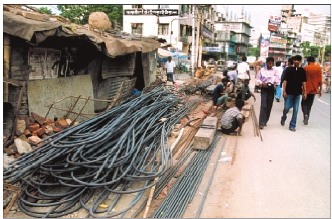
Tangled rods and building materials kept on the stretch of road near Baitul Mukarram National Mosque opposite the National Sports Council in Purana Paltan yesterday speak of the developer's apathy to obstruction to public movement.
