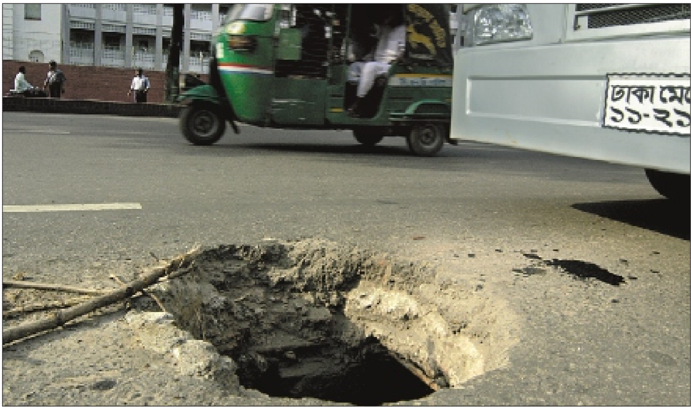
An open manhole threatens traffic movement on Abdul Ghani Road in front of the secretariat that houses most government offices.
