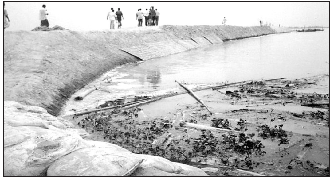
Nilkuthi cross dam being build by local people is threatened by Jamuna water.
