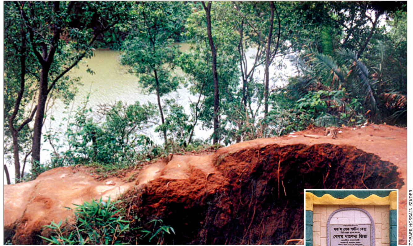
Foy's Lake: A huge chunk of earth has collapsed at a hillock by Foy's Lake during the first shower of the season recently. It reminds the necessity of immediate start of the project taken up for developing Foy's Lake park-cum-amusement centre to attract more tourists. Prime Minister Khaleda Zia laid the foundation stone of Foy's Lake Tourism Centre at Pahartoli on April 19.
