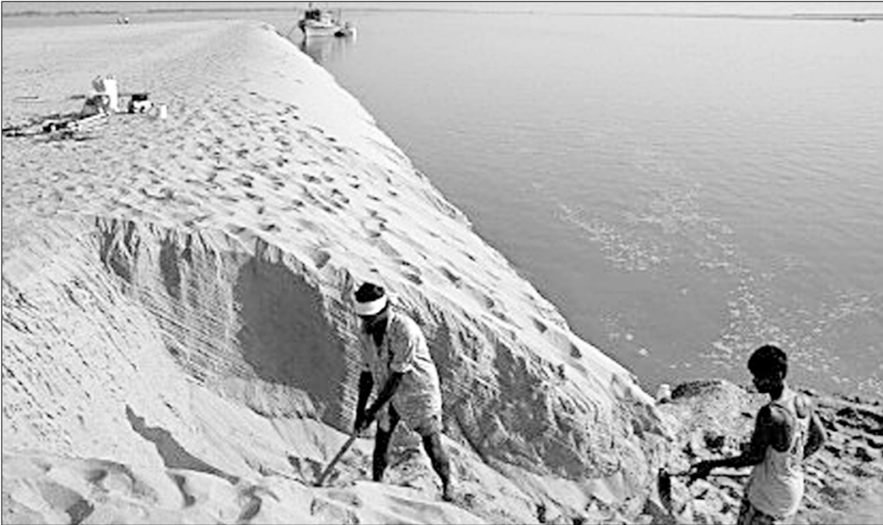
Workers are seen at a construction site for a dam or river project.
