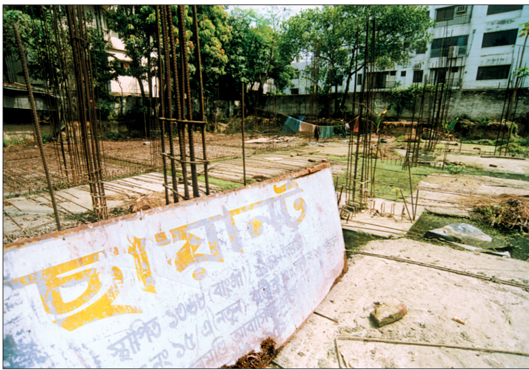
Construction work of Chhayanaut Bhaban remains suspended for not following Rajuk code.
