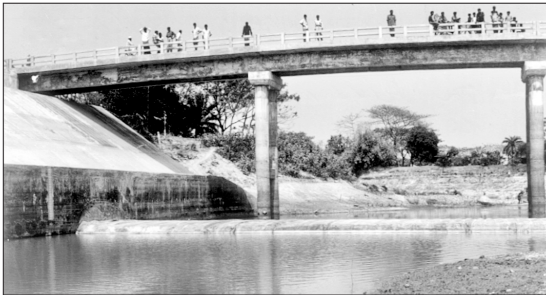
A faulty rubber dam built at Urahati point on the Khiru in Bhaluka, Mymensingh.
