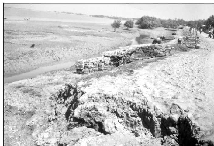
Earth has been removed from WDB dam at Khalishabunia. Brick, cement and sand have been piled up for construction of a sluice gate there.
