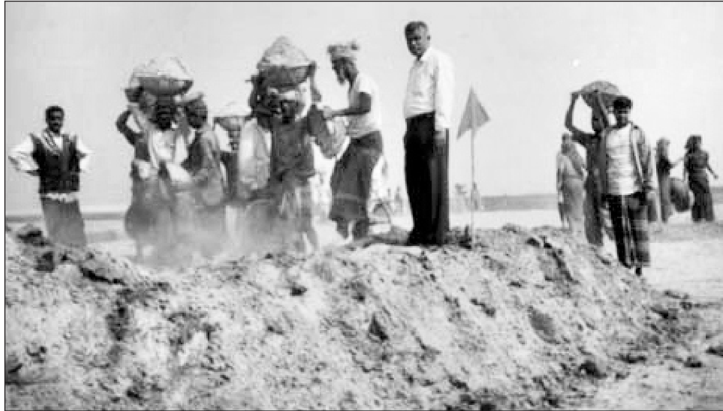
United they stand and do a great work...men and women from all classes building a dam to protect the Fulchhari upazila headquarters.
