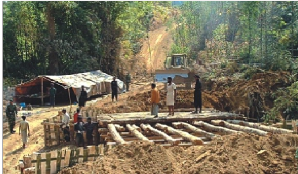
A bulldozer clears trees to make way for the road to Sajek. An army team supervises the work to connect the remote union to Khagrachhari town.
