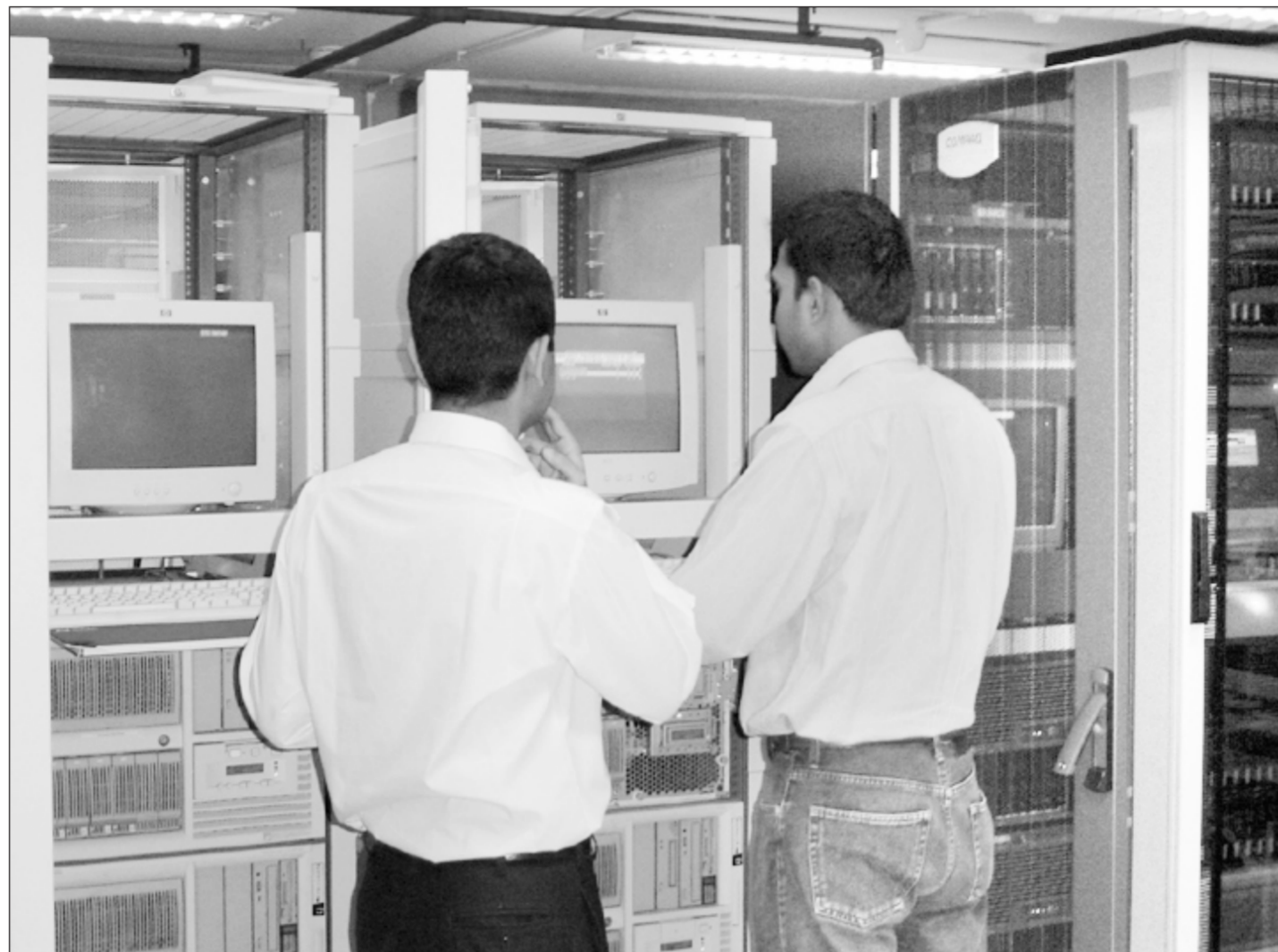
The newly installed system provides enhanced security, smoother operation and maintenance capability of the system and user level access control
