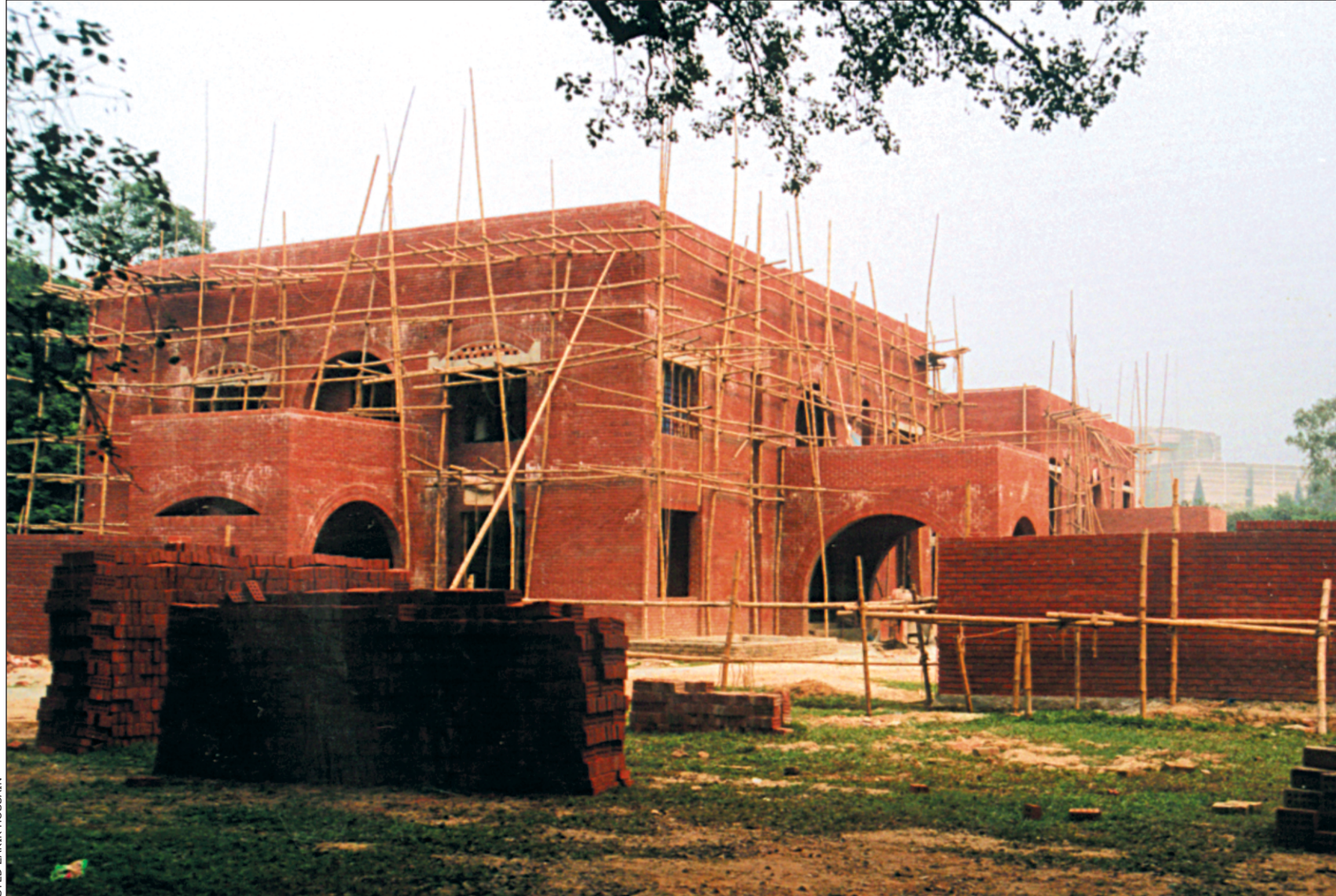
The speaker and his deputy's houses inside the parliament complex will be complete by March: Nobody to speak out?
