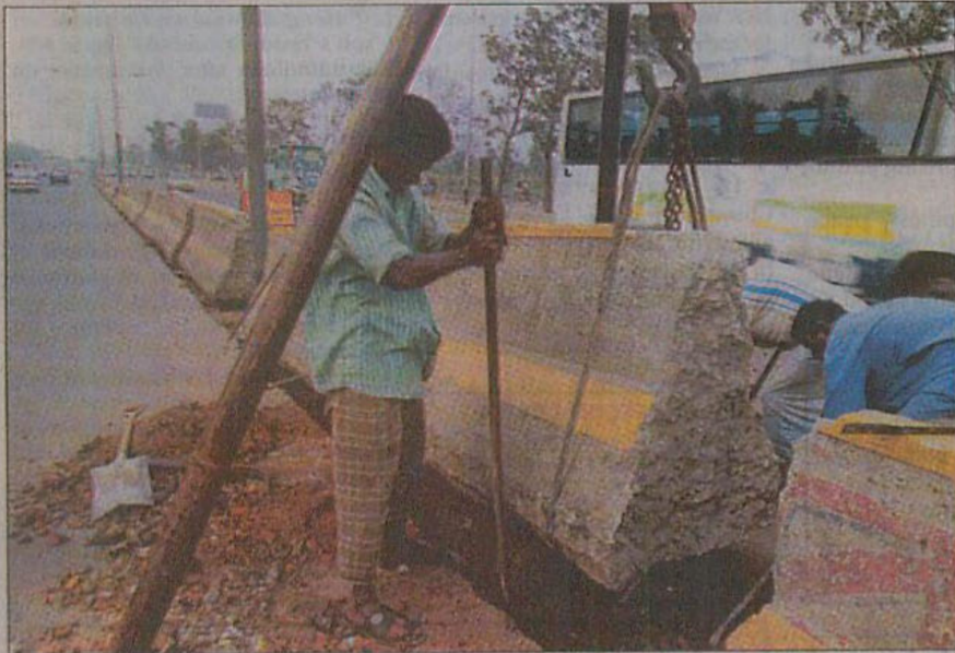
Roads and Highways Department workers replace concrete blocks to reconstruct the road divider on Airport Road yesterday.
