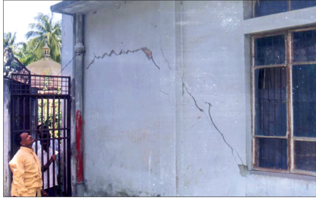
Morning jolts leave buildings in cracks in the second largest tremor since 1997 that also left 25 people injured in Chittagong yesterday.
