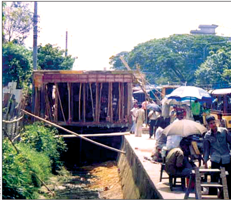
Construction is going on for extension of a bus terminal (Rangamati, Khagrachhari) on a drain beside busy Muradpur road in the city.
