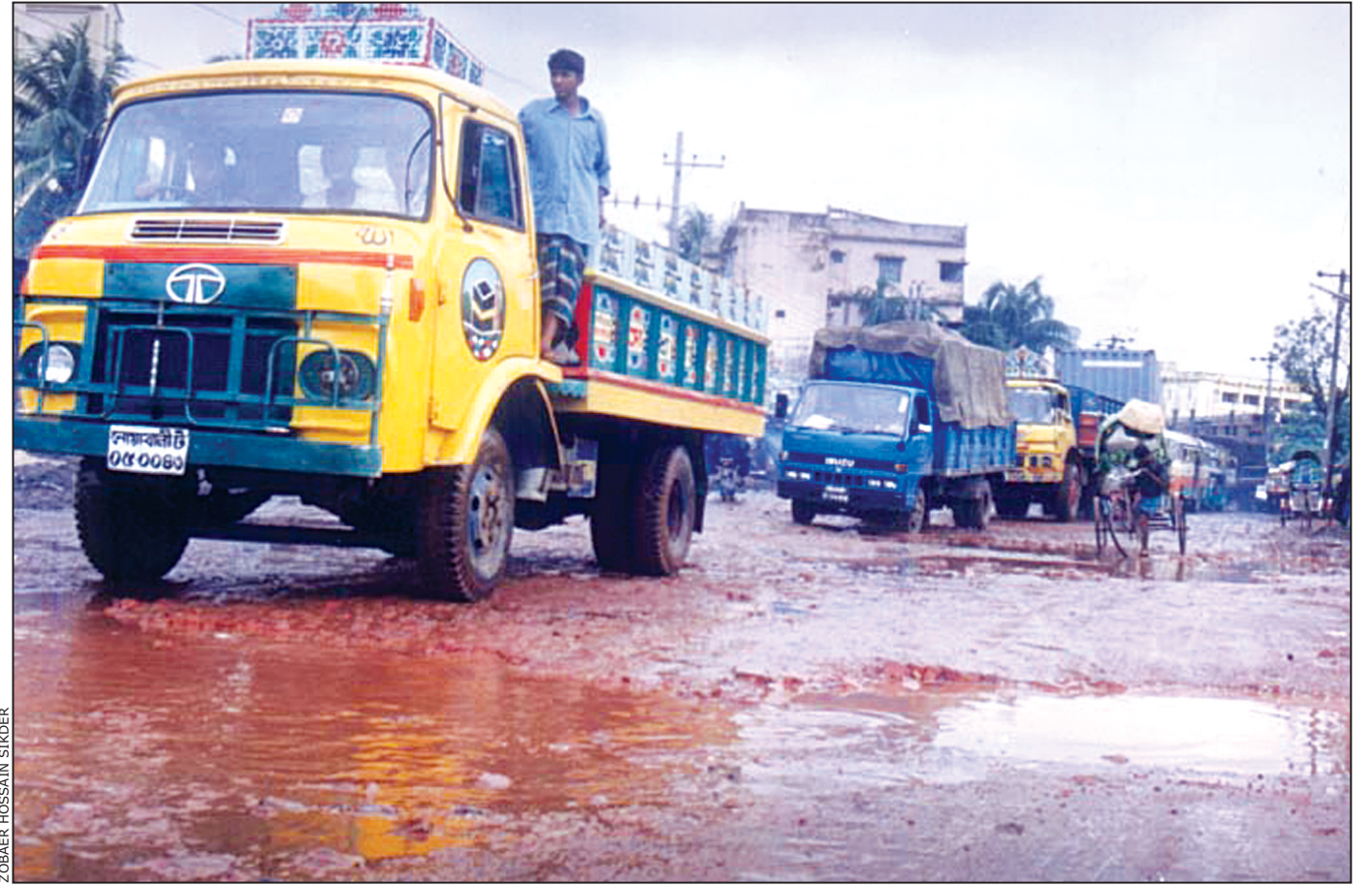
Dilapidated Arakan Sarak (Chittagong-Cox's Bazar highway) on both sides of Kalurghat bridge causes hazardous traffic movement.
