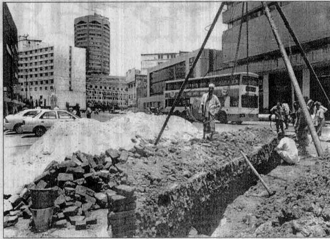
Fresh road-digging at Motijheel bears testimony to the lack of coordination among different government agencies. The drainage department of WASA has dug up a part of the road at Motijheel although it has been repaired recently.
