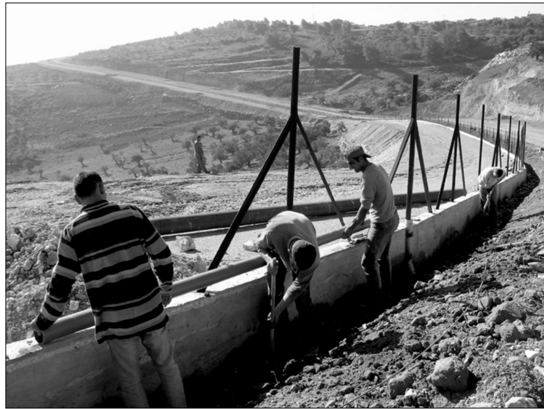
Workers build the separation fence between Umm Al-Fahm in northern Israel and Anin in the Palestinian West Bank on Sunday. After two years of conflict, the Israeli government launched the construction of a 350-kilometre security fence which loosely follows the Green Line in a bid to prevent Palestinian militants from infiltrating into Israel.
