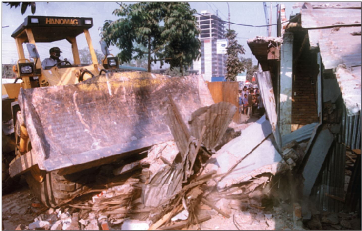
The Bangladesh Railway razes illegal structures to the ground in a cleanup drive on both sides of a railway crossing on Sonargaon Hotel Road in the city yesterday.
