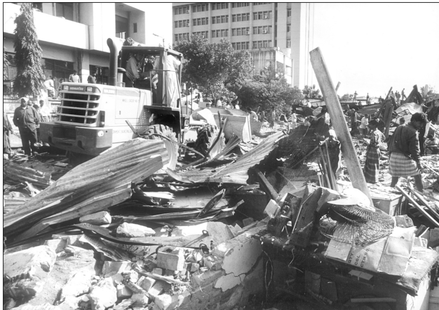
Rajuk runs a cleanup drive in which about 500 illegal structures were razed to the ground behind the Local Government Engineering Department (LGED) building at Agargaon in the city yesterday.
