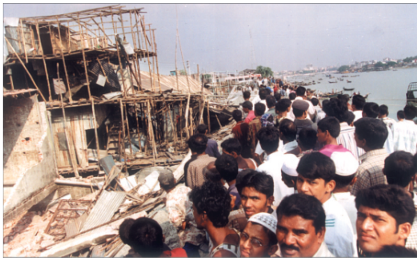
Curious people look at pulled-down structures on the foreshore of the Buriganga near the city's Muslimbagh area yesterday, the fourth day of the Bangladesh Inland Water Transport Authority (BIWTA) anti-encroachment drive.
