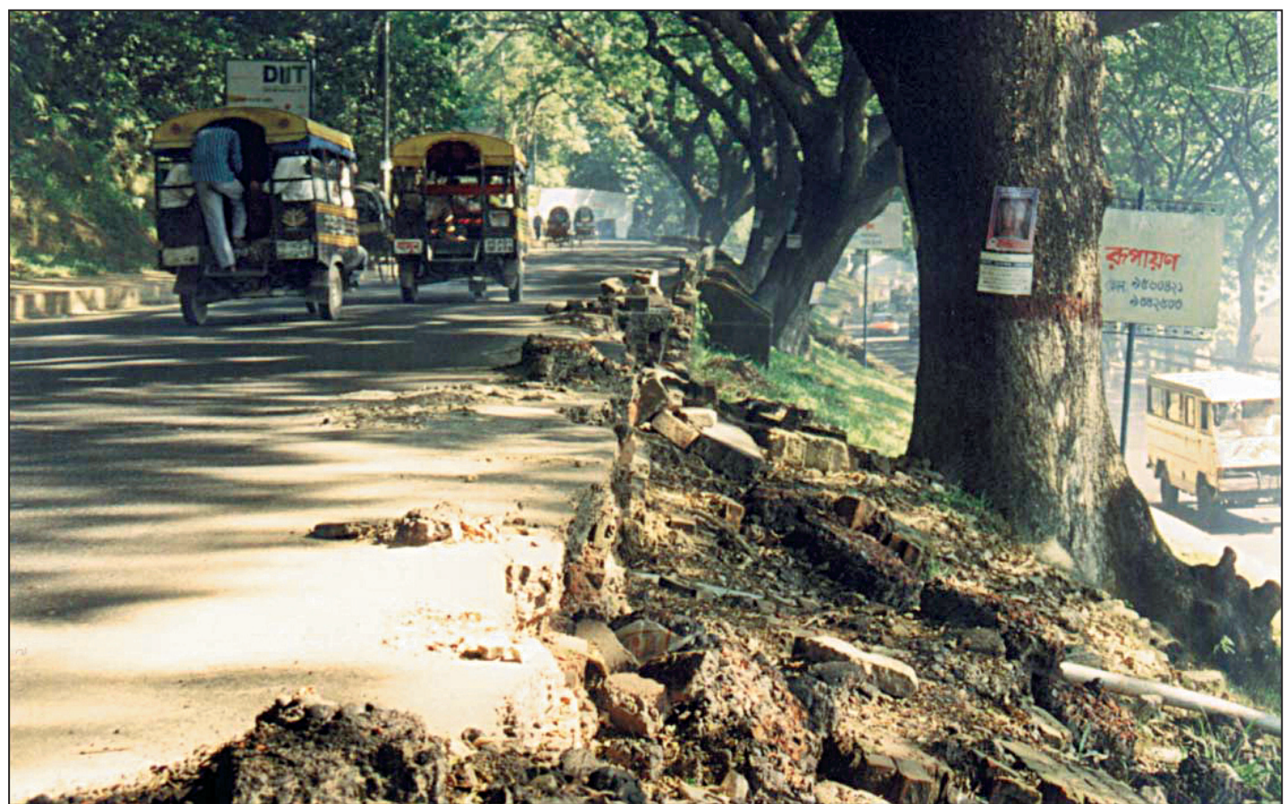
A portion of the wall on the road at Pologround area near Tigerpass intersection collapsed, threatening vehicular movement.
