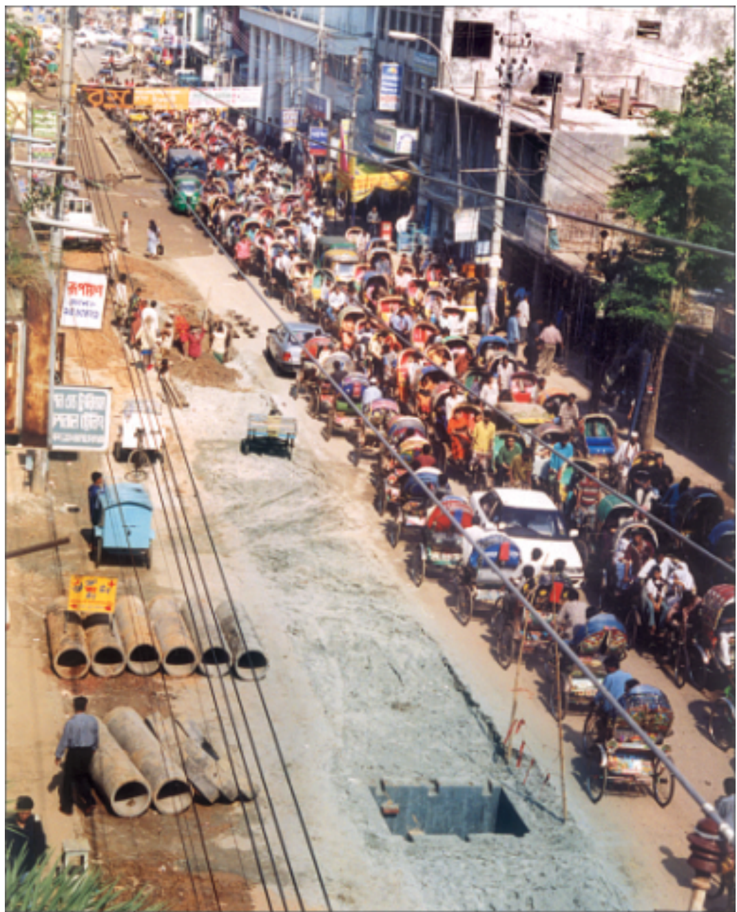
Hundreds of rickshaws and some other vehicles are stuck in a traffic jam yesterday on the city's Green Road that has shrunk to a narrow stretch due to digging.
