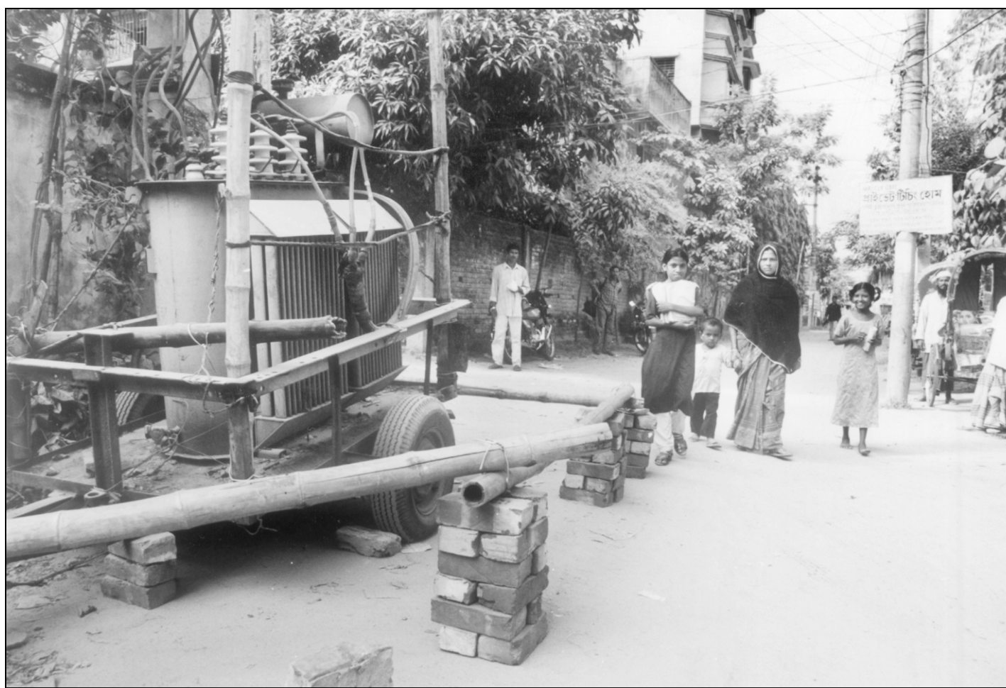
A schoolgirl passes by a power transformer on a road in the city's Mohammadpur yesterday. The transformer, set up without any precautionary measure, may cause serious accident any time.
