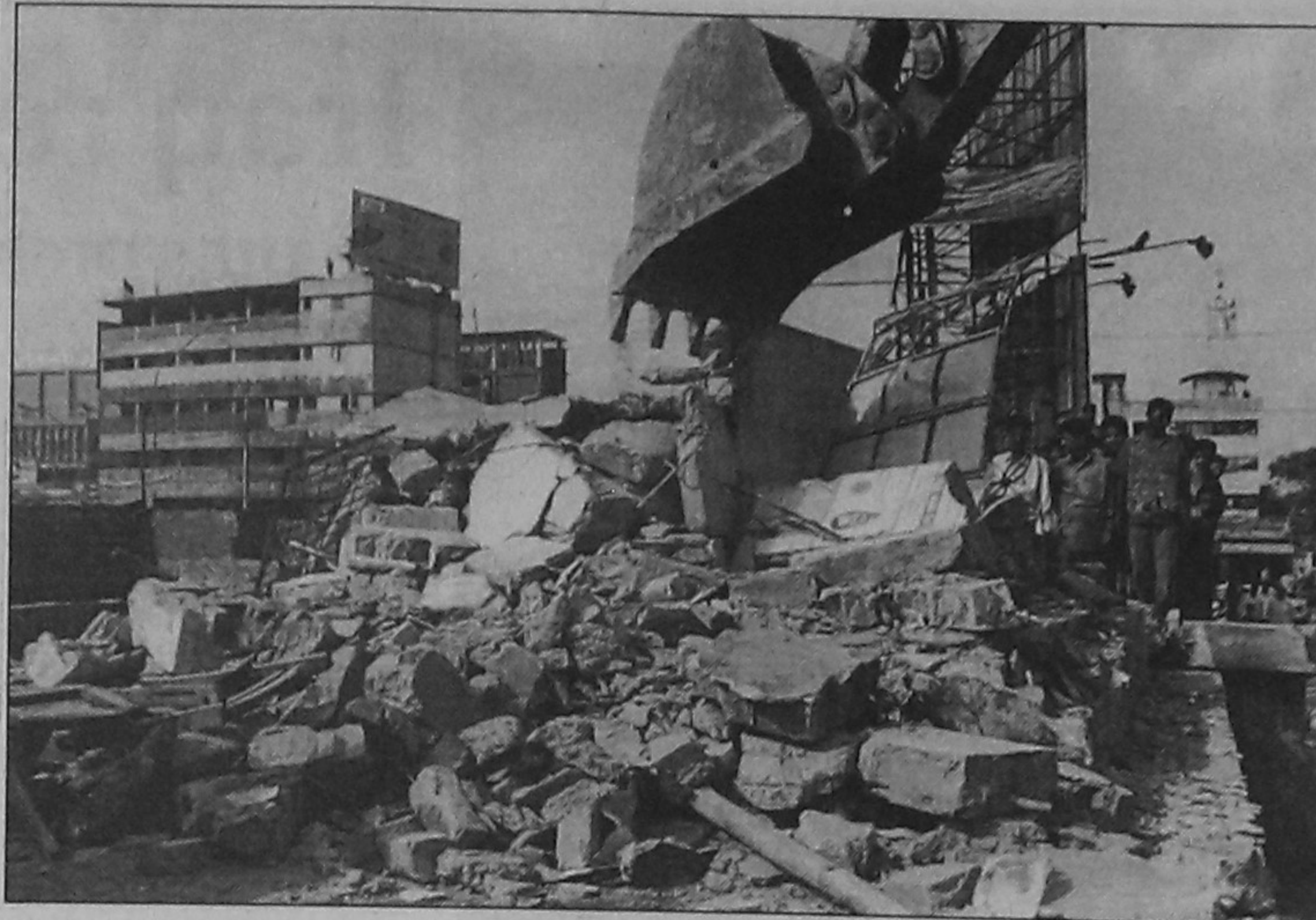
The Water Development Board demolishes unauthorised structures near embankment at Rayer Bazar in the city yesterday.
