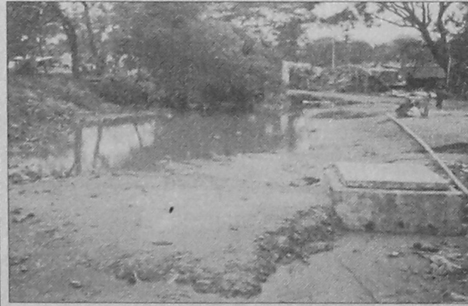
Because of unauthorised filling of a canal of the Roads and Highways (R&H) department by some influential, water remains stagnant for days together on the South Surma Bus Terminal road in Sylhet. Influentials here have been grabbing government lands illegally for a long time, but the authorities concerned are still indifferent to recover the lands.
