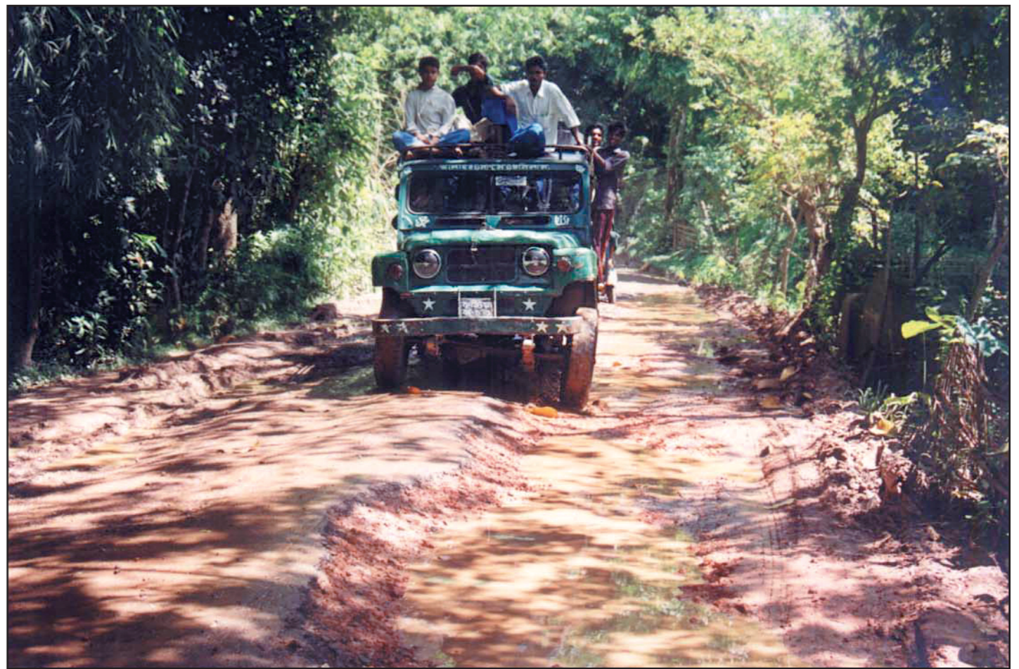
A three kilometre stretch of Fatikchhari-Haiyanko road remains in a dilapidated condition for long posing a great risk to vehicular movement.
