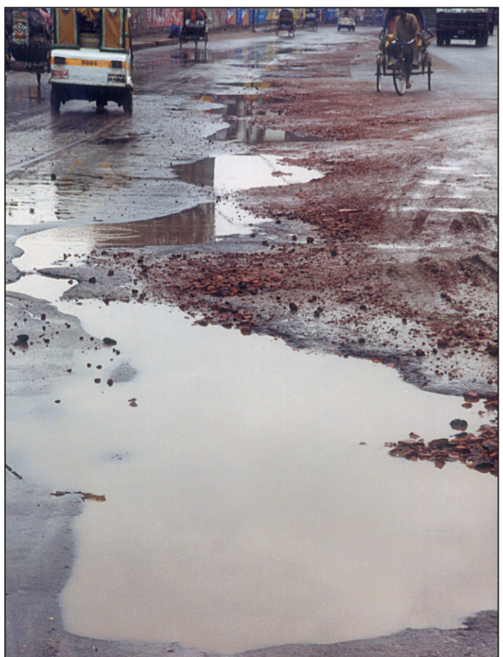
The pothole-strewn Bashabo-Khilgaon-Sayedabad Road is no longer safe for traffic. Unfortunately, the longstanding problem failed to draw attention from the Dhaka City Corporation (DCC).
