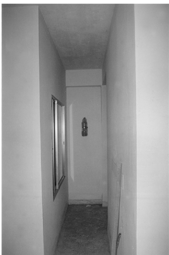
Fig. 5: Western Tower Apartment: A narrow passage of 2'-6" width provides access to the fire exit with the only fire extinguisher located at the dead end corner.
