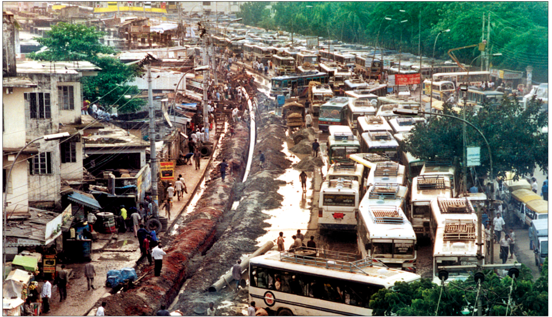
City of nightmare...a long queue of buses crawl at a snail's pace through the road between Joy Ma Kali temple and Gulistan yesterday as the road digging by the Titas gas authorities to lay pipelines has caused a havoc to traffic movement.
