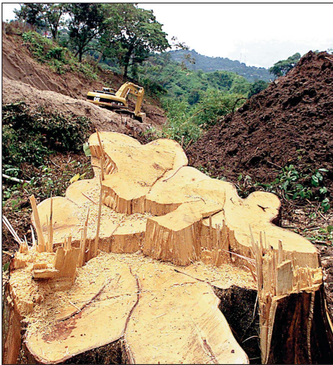
An excavating machine digs up earth on a road under construction near Ciudad Delgado, El Salvador on Wednesday. Trees are also falling victim to construction as residents of the area and ecologist protest to stop the work, pointing that the destruction of the trees will affect the area's ecosystem.
