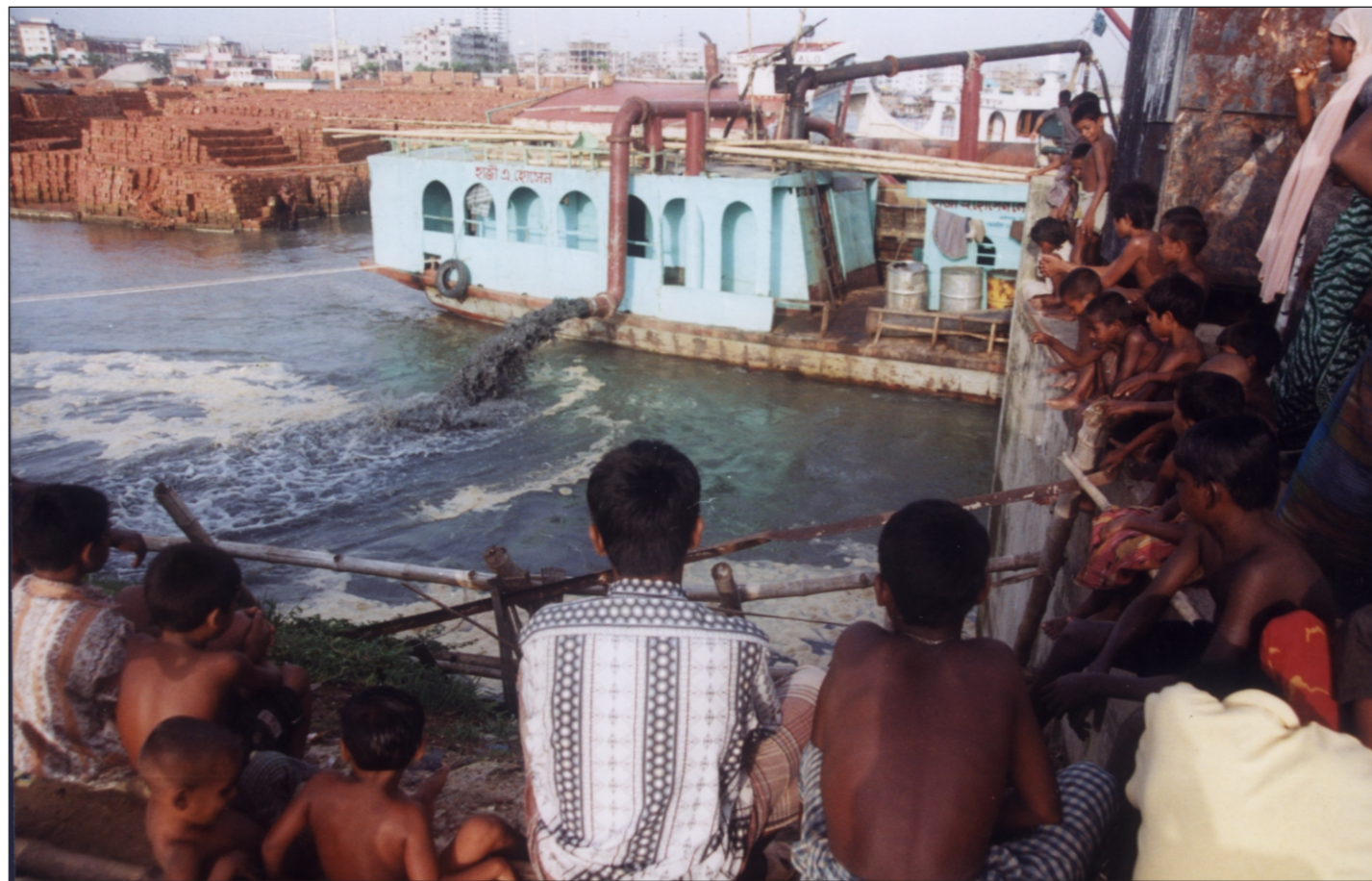
Witness to mindless action... A dredger operates to fill up the Haikkar Khal near the martyred intellectuals' monument at Rayer Bazar to build a truck terminal there.
